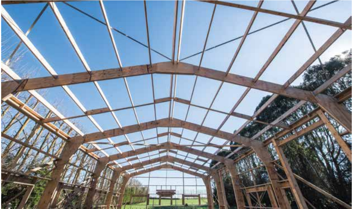
Large Futurebuild® LVL hySPAN columns and beams enabled a 4.2m clear span.
